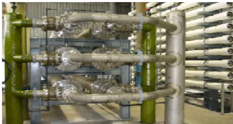
SAF 2507 duplex stainless steel (3-5% Mo) piping in a reverse osmosis desalination plant.
