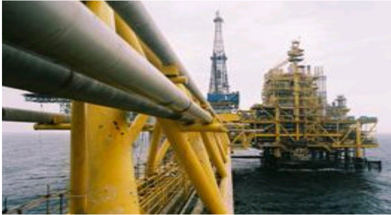
254 SMO (6% Mo) pipes running to an offshore Qatari platform, itself rich in austenitic and duplex stainless steels containing molybdenum. (Source: Maersk Oil)
