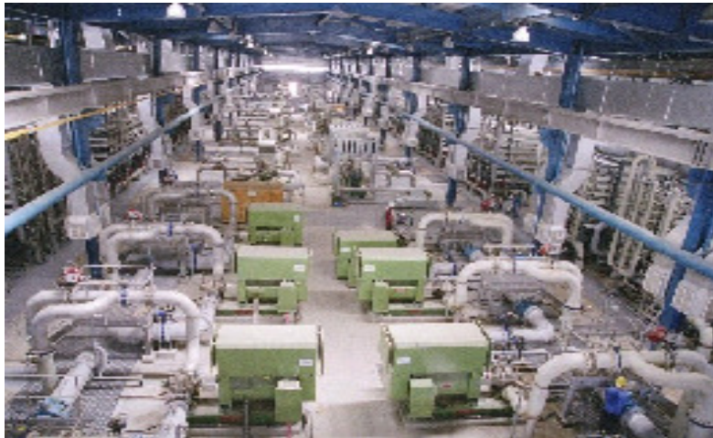
Fujairah, United Arab Emirates, desalination plant showing 254 SMO (6% Mo) high-pressure piping.
