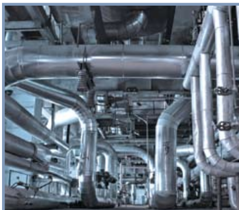
Pipes inside a nuclear power plant
